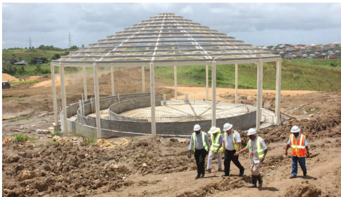
On one of his regular visits to the site of the South campus of The UWI, Principal of the St Augustine Campus, Professor Clement Sankat walks past the framework for the Moot Court, part of the Faculty of Law, with members of the construction and campus teams. The new Dean of the Faculty of Law, Professor Rose-Marie Belle Antoine's appointment took effect earlier this month. She replaced Dr Kusha Haraksingh, who held the post as interim Dean for one year. PHOTO: ANEEL KARIM
