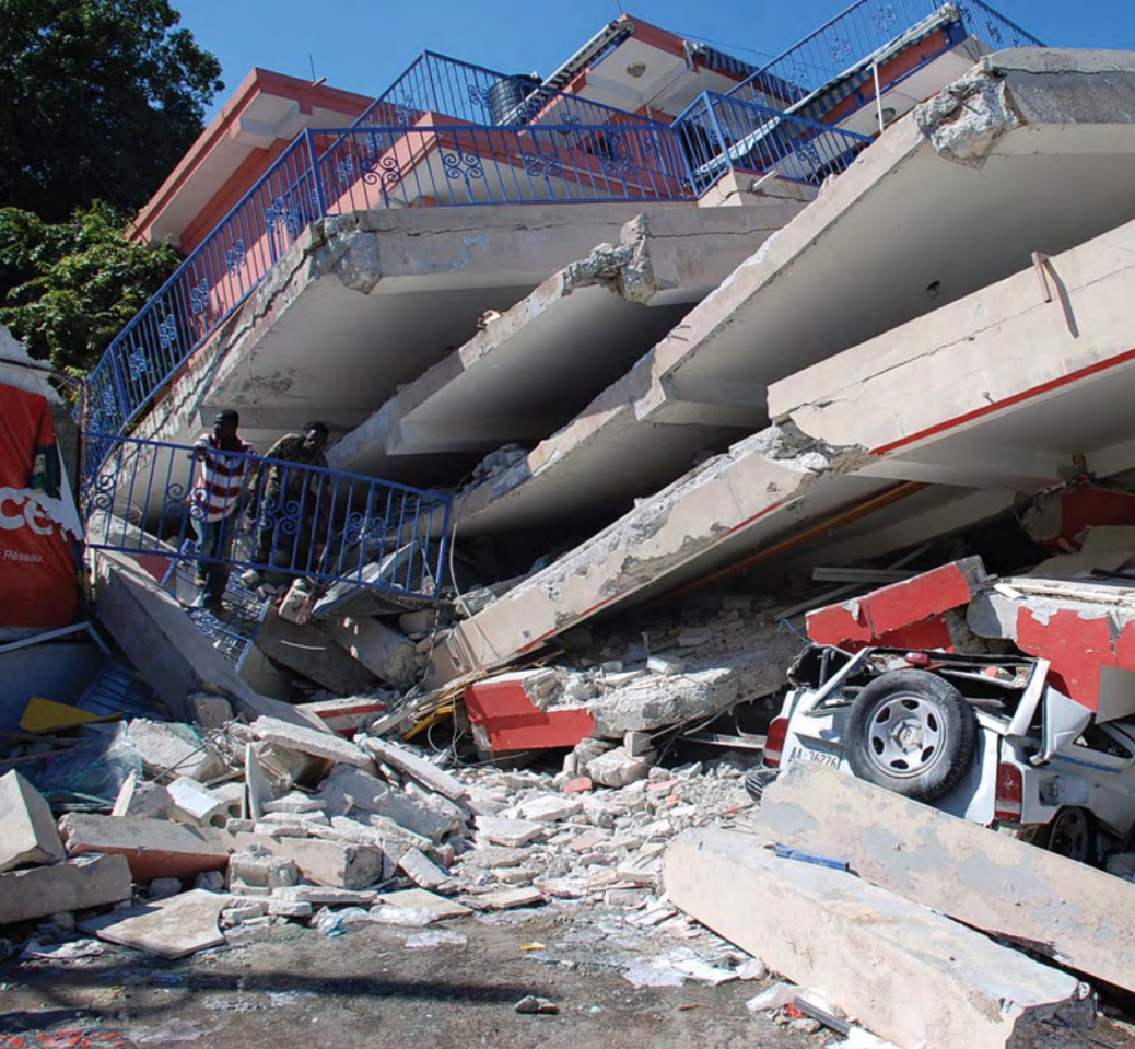
Force of nature added to poor structure = flattened building. (photo by Eric Quintero)
