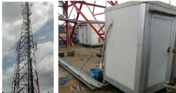
Figure 2. Pictorial view of a typical eNodeB site located in Ajah area of Lagos, Nigeria
