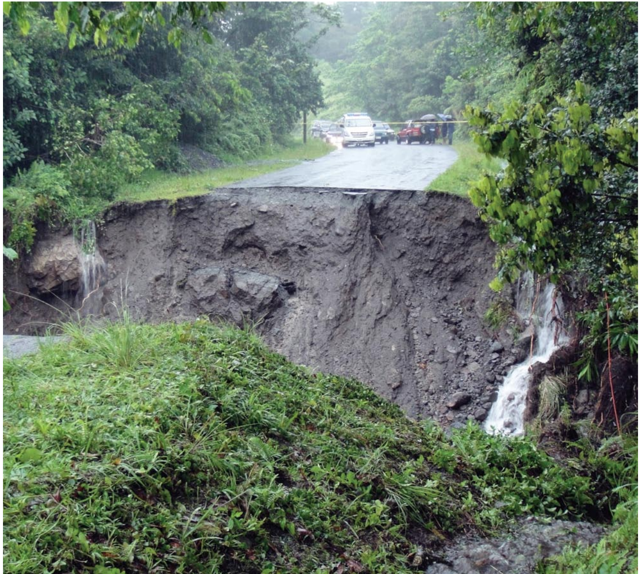
Road Failure at Pont Cassé PHOTO COURTESY: CHIEF TECHNICAL OFFICER, MINISTRY OF WORKS, GOVERNMENT OF DOMINICA
